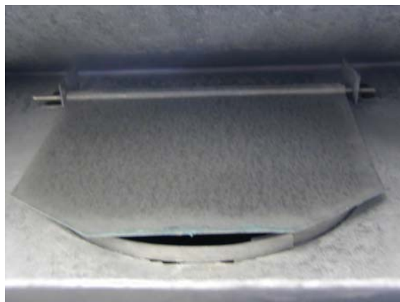
Fig. 11B Improperly closed backdraft flapper
