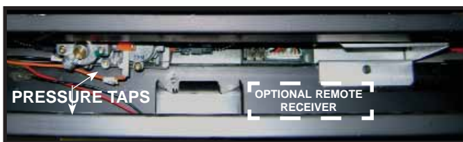
Figure 11.5 Valve Pressure Taps and Remote Receiver Location
